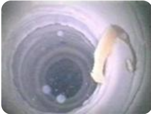
Filter recirculation pipe with sodium hypo
