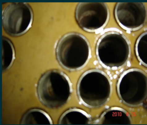
(June 2010) U15 Main Condenser Tube Sheet after extended run – before cleaning, after 2.5 Months of MIOX treatment
