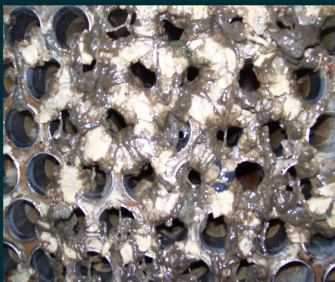
(June 2008) U15 Main Condenser Tube Sheet after extended run – before cleaning, after non- MIOX treatment
